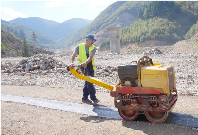
Physical construction works of Plovdivtsi Dam wall were completed and the reservoir has begun taking on water.
